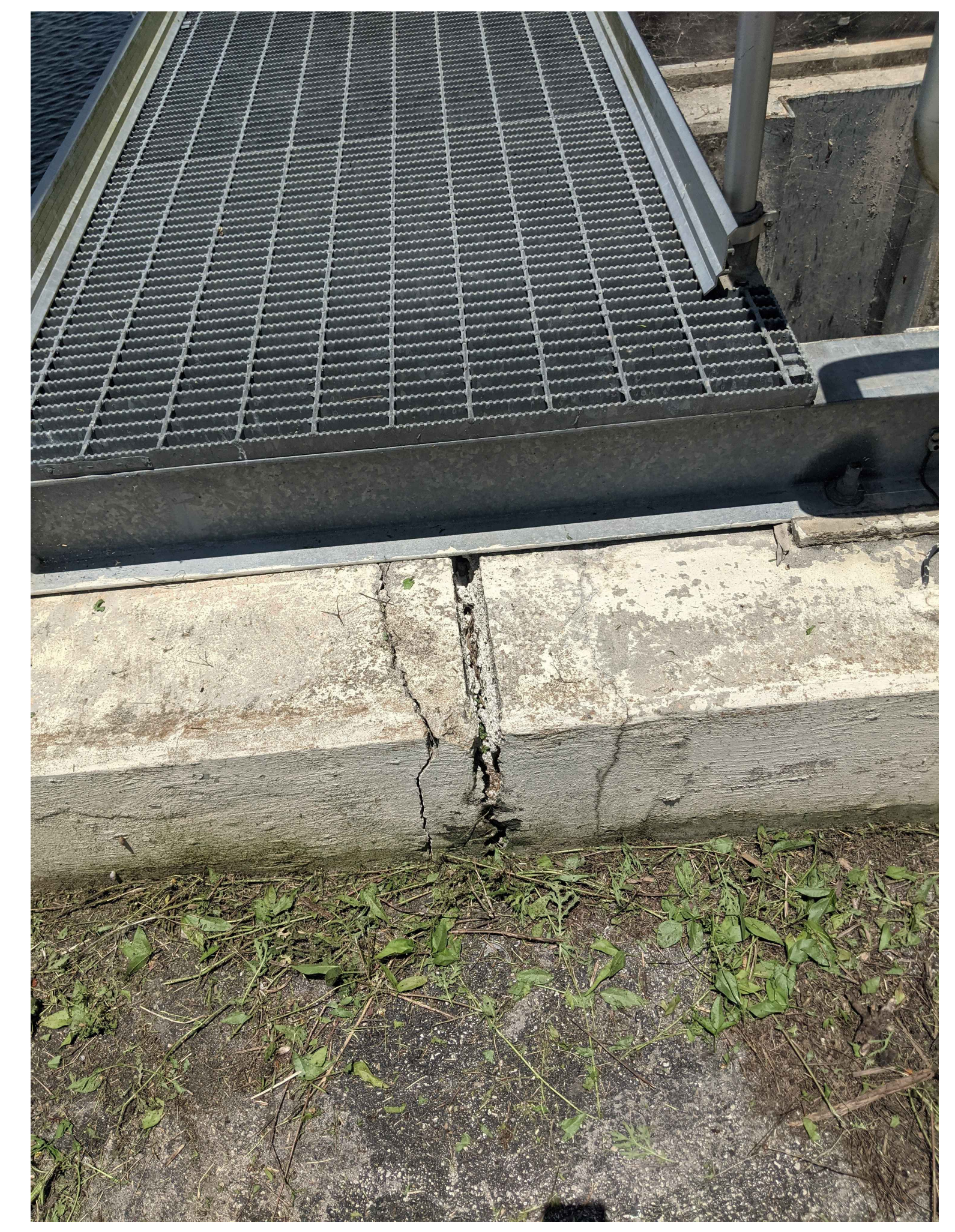
CRACKING AT G-372 CONCRETE PILE CAP
