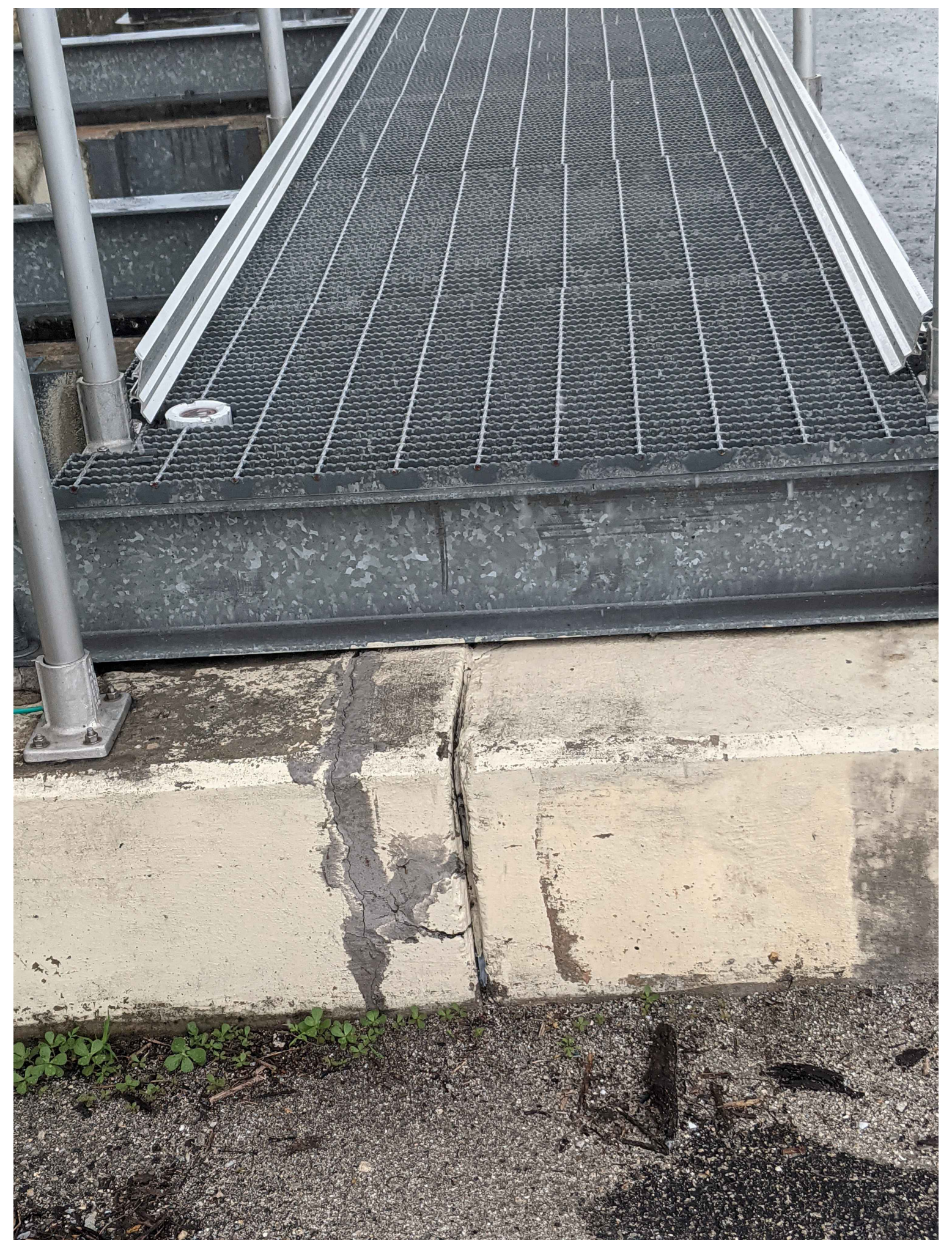
CRACKING AT G-370 CONCRETE PILE CAP
